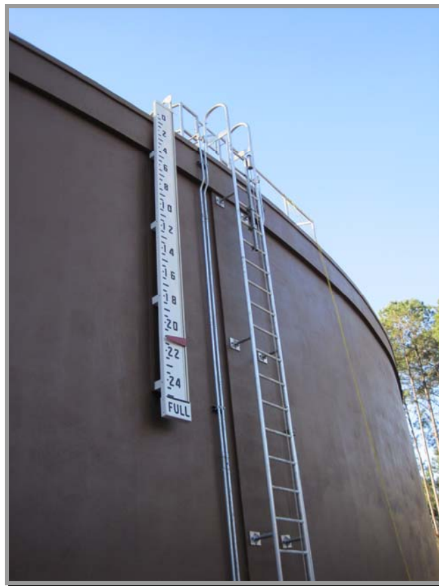
ASR3 tank level indicator and ladder
