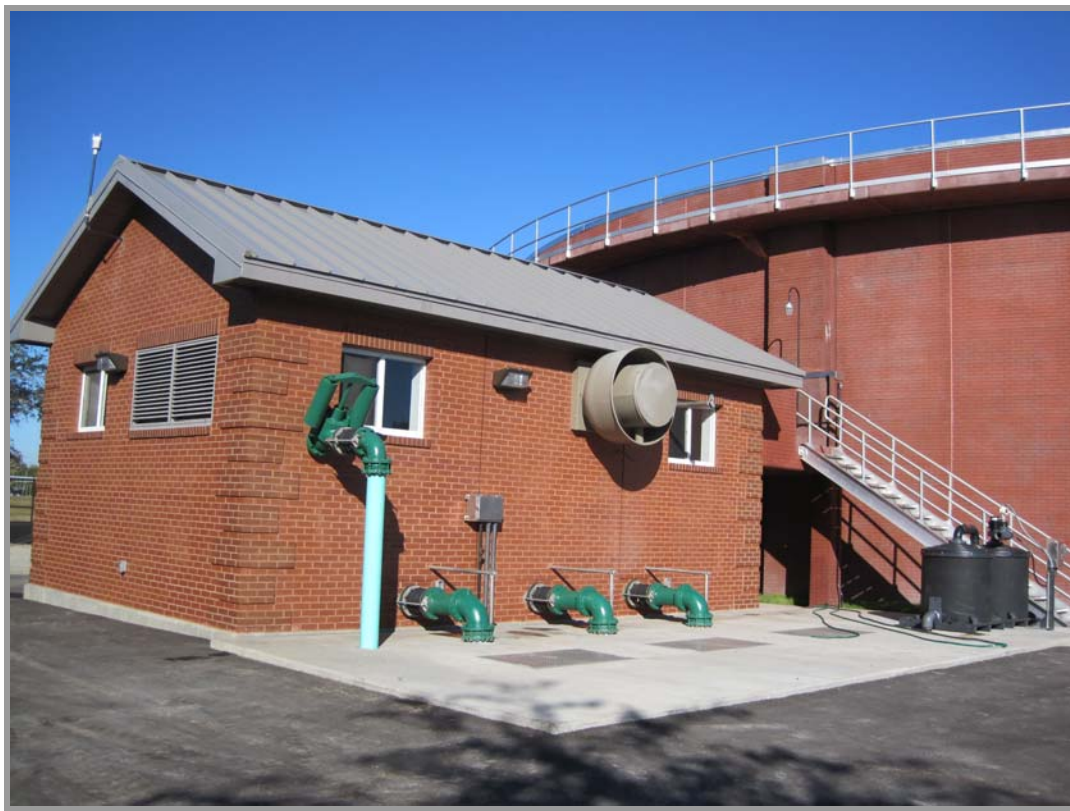
Parris Island Pump Station and Tank
